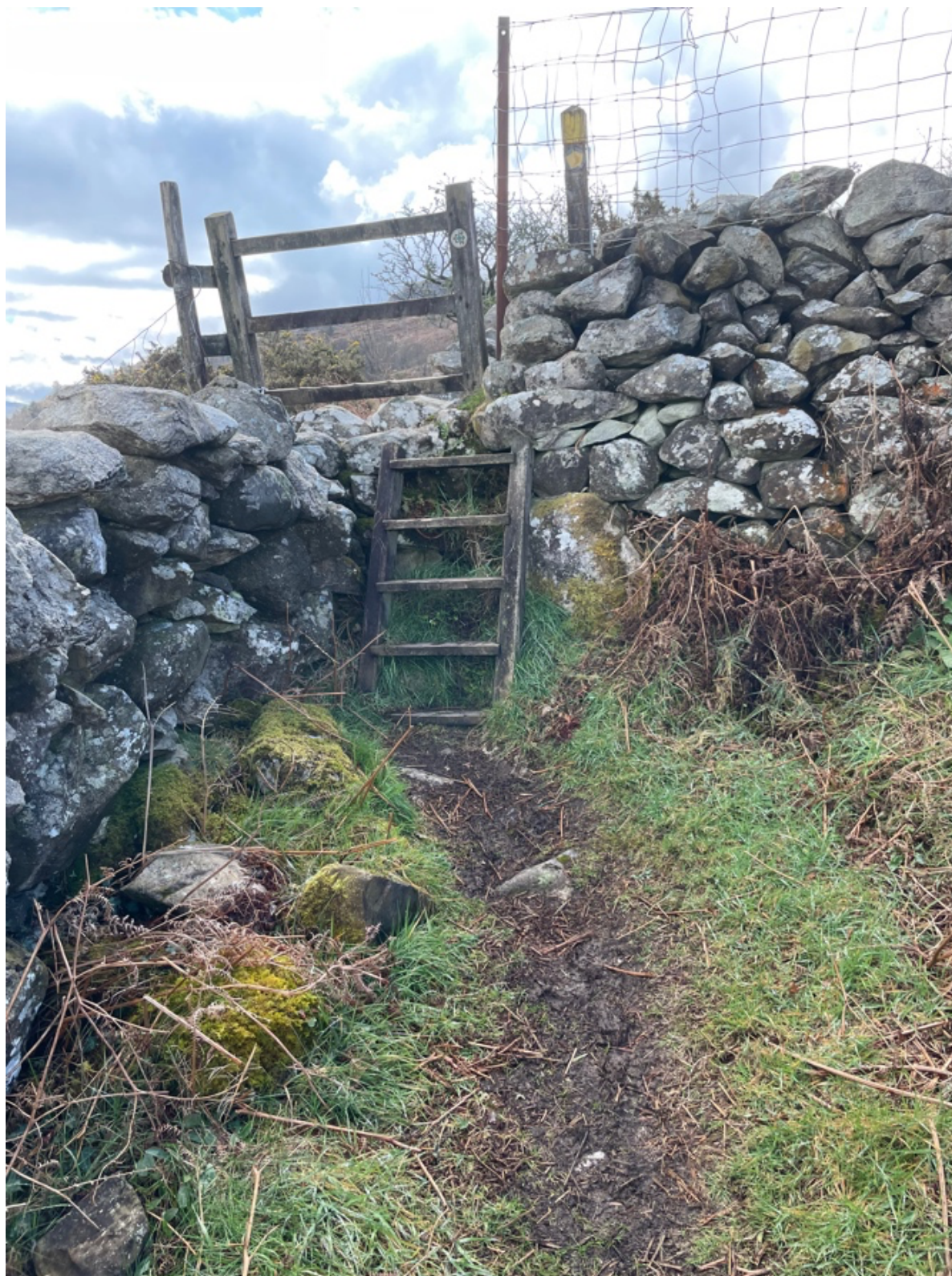
Photo 65 – precarious ladder stile /railing northern edge of woodland out of Waunfawr which is exposed and tricky to use especially as at height in stone wall corner with drops either side - could do with safer structure over. SH52076 58385.
